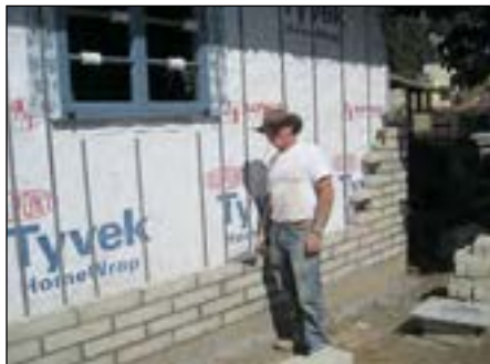
Willie Quinn, masonry sub-contractor, building a jacket of concrete blocks around the exterior walls of the new library extension.
