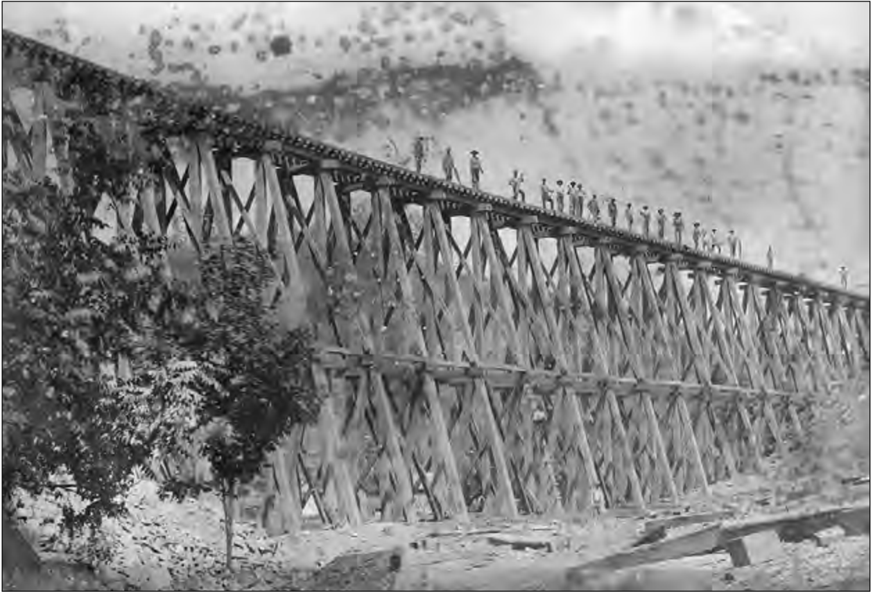
Tintype of a railroad crew building a bridge. It is not known if it was William McDuffie's crew.
